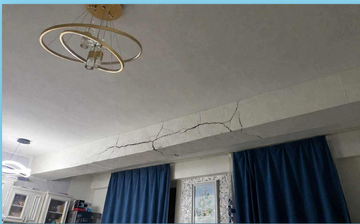
Figure 5. Cracks in Building No. 208 caused by the earthquake.
