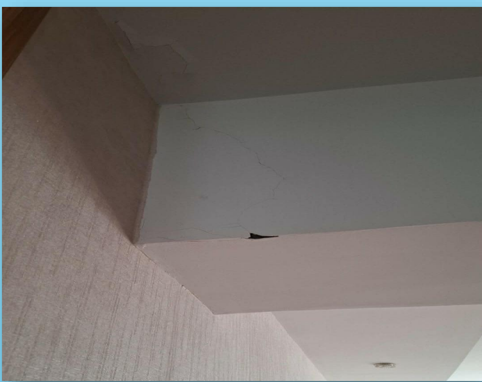
Figure 6. Cracks in Building No. 104 caused by the earthquake.
