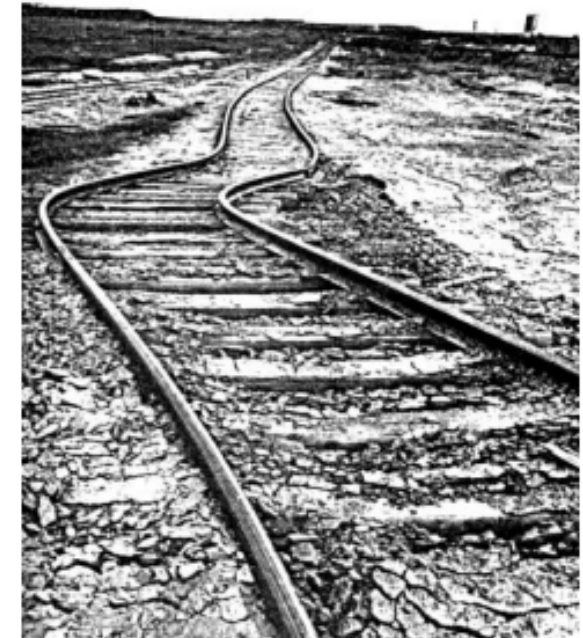
deformation of the rail track
